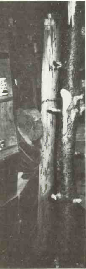
Wall begins pushing in due to poor engineering. Post at right (bark on) is an emergency support.
